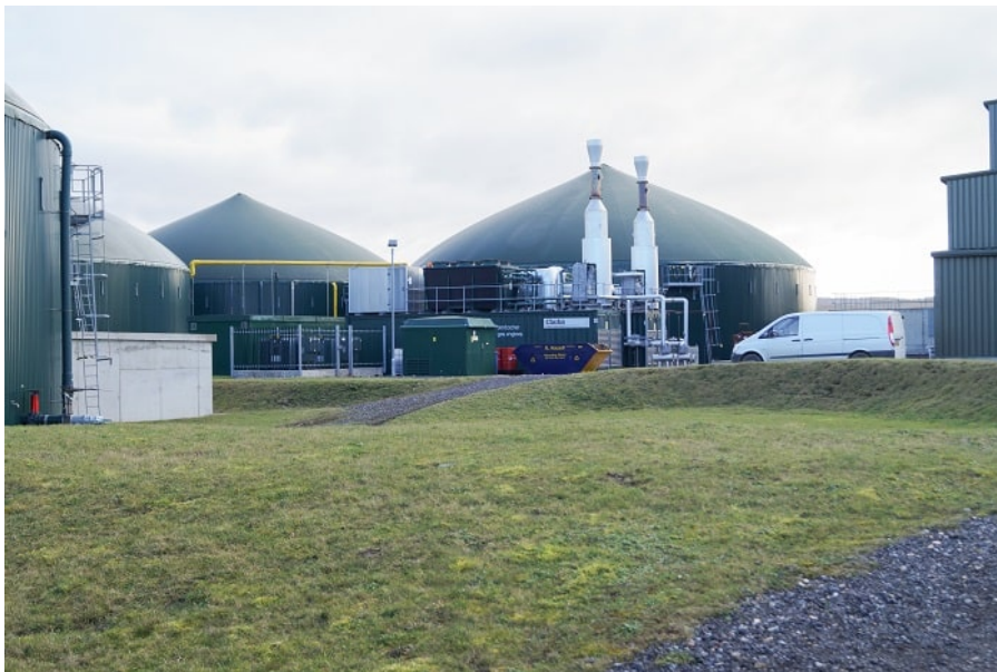
Agrivert's Wallingford anaerobic digestion facility
